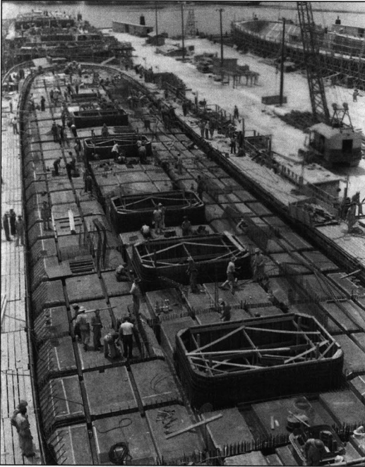
Despite wartime labor shortages, most jobsites remained male-dominated. Here, a civilian crew builds a reinforced concrete ship at the Mallory Docks in Tampa, 1943-44. (Photograph courtesy of the Tampa Historical Society.)
